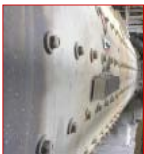
Peltier power supply mounted on mill shell
